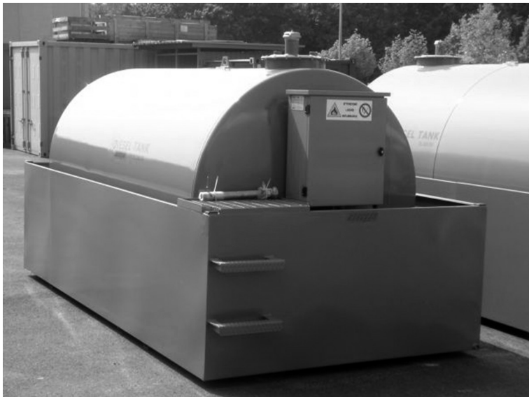
Picture 5. Mobile safety bund. [10]
