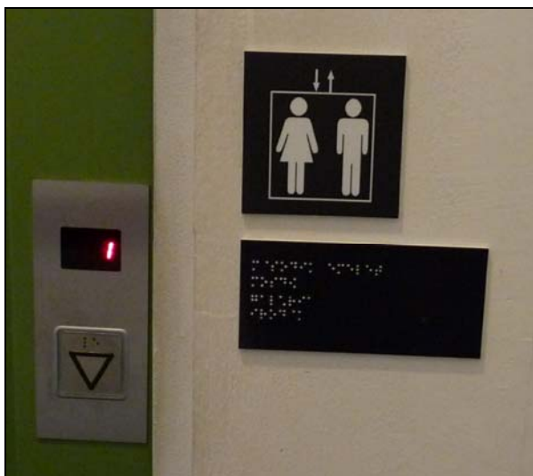
4. ábra Lift panel
