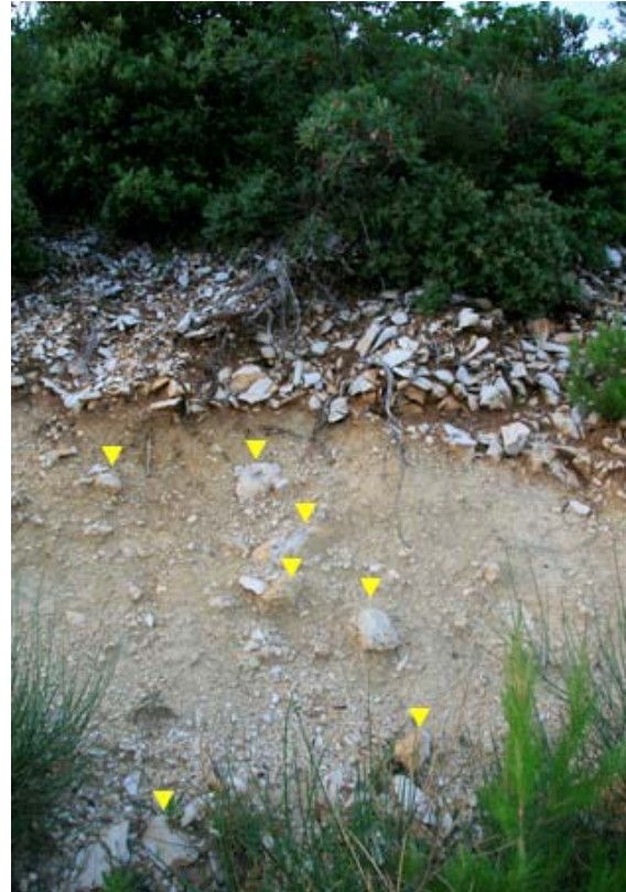
Fig. 6.: Fire access road cut section with eroded chert. Matetina Peć, Kozjak Mountain
